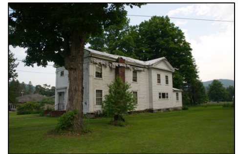
Above (top to bottom): A Classic Greek Revival home on Second Street in need of repainting and other repairs; another example of a Greek Revival home, this time showing a home that is in a serious state of disrepair with a leaking roof, loss of front porch overhand and neglected exterior. When historic properties are allowed to become dilapidated they diminish property values, while these same homes restored would dramatically increase property values in the Village.
