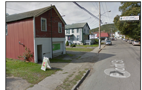
Above (top to bottom): Culvert crossing the Butler Brook at the corner of Division Street and Front Street that needs to be replaced (sidewalk is closed and weight limit posted); view of some segments of paving along Front Street that are beginning to crack and need to be sealed, and view of curbing, sidewalk and drainage deficiencies near the Front Street-Elm Street intersection. This Plan supports Village grant applications to secure funding to address these deficiencies.
